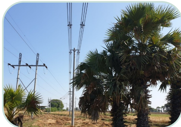
6.6kV Overhead Transmission Line
