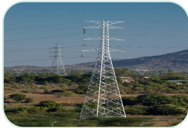
230 kV Transmission Tower
