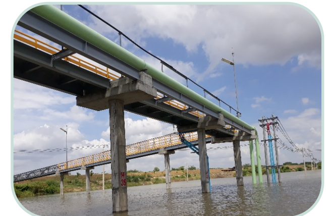
Water Pipeline (Intake & Discharge)
